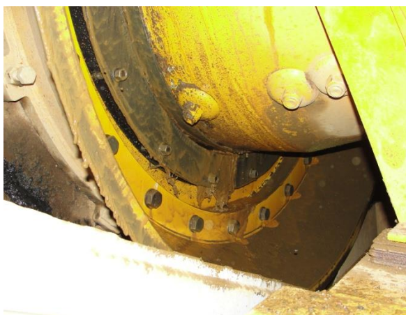
Figure 8 Slurry spilling from the mill feed end
